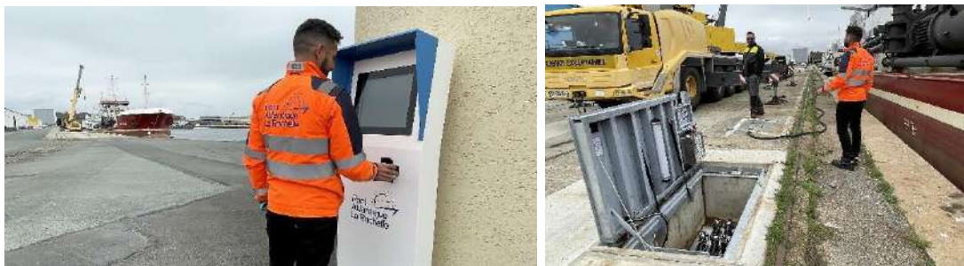
Figure 27 : Electrification des quais
